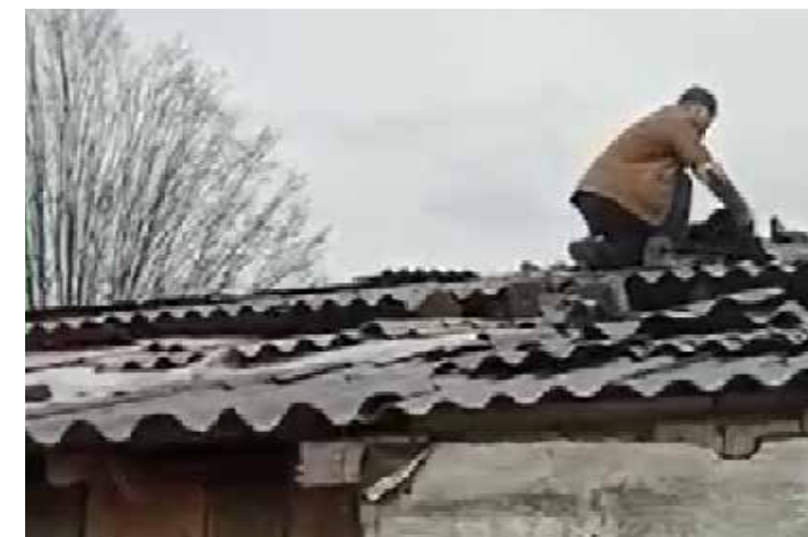
Igor works to cover the leaking roof.
